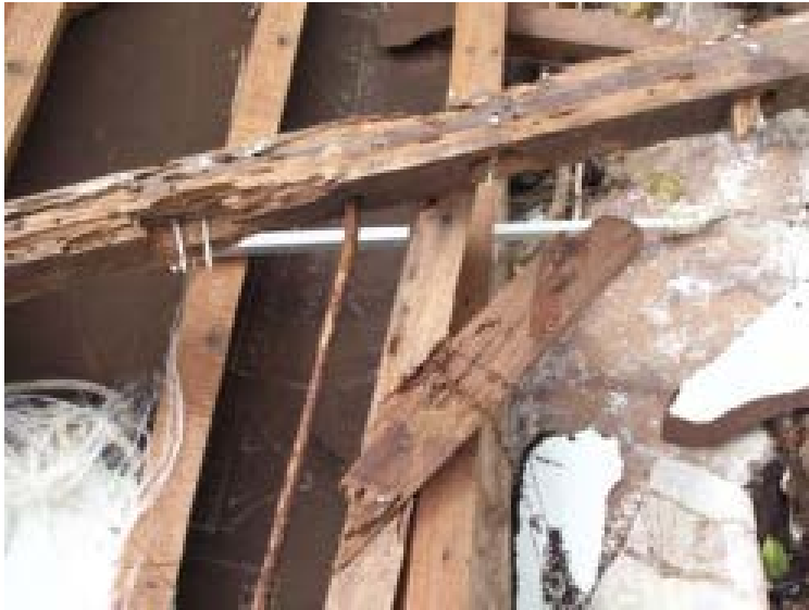
Termite attack to timber
