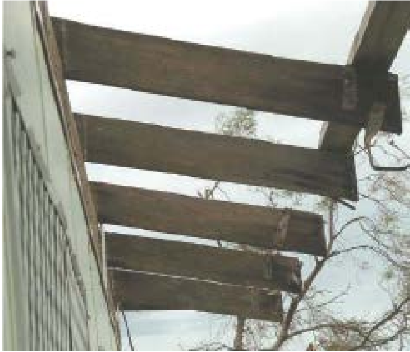
Corroded batten straps contributing to roof failure
