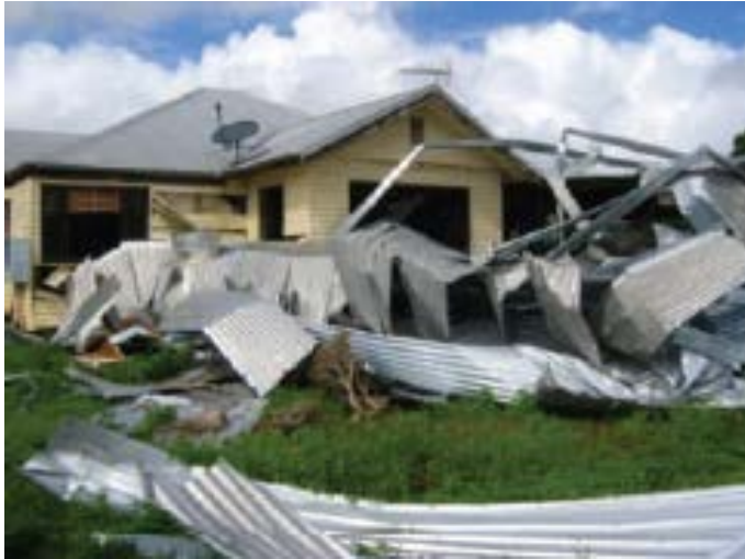
Flying debris resting in front of a house
