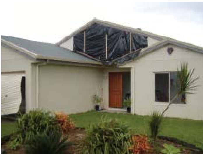
Failure of a gable end wall allowing strong wind and rainwater into the house
