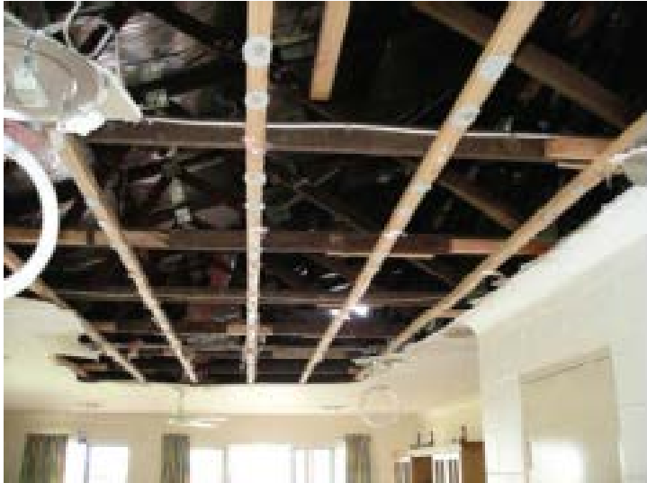
Damage to ceiling due to water ingress
