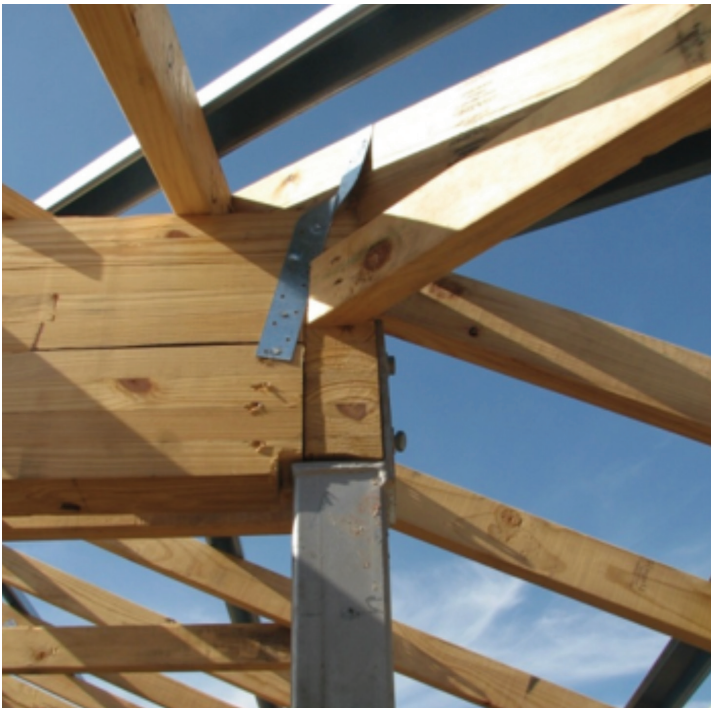
Photograph 16 – Intersecting verandah beams. The LH beam has inadequate bearing and tie-down capacity
