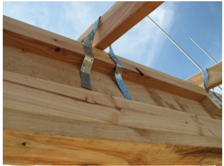
Photograph 10 – Truss tied direct to top plate and lintel, but strap bent through too great an angle to be effective
