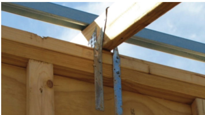
Photograph 1 - Inappropriate practices as nails are too close to strap edge, too close to pre-punched holes and even doubled up. Strap should also have been installed on the inside of frame to enable strap nailing direct to lintel without bending the strap
