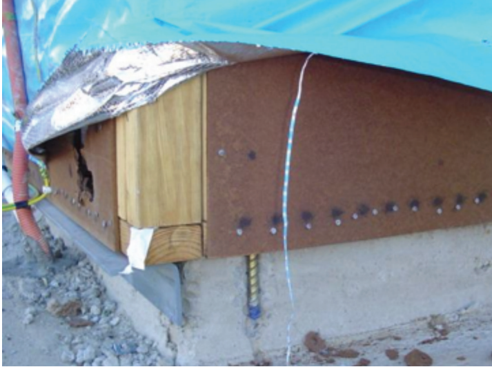
Photograph 12 – Structural integrity totally compromised by excessive bottom plate overhangs
