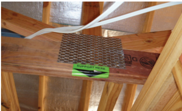
Photograph 6 – Girder truss incorrectly supported by an offset wall
