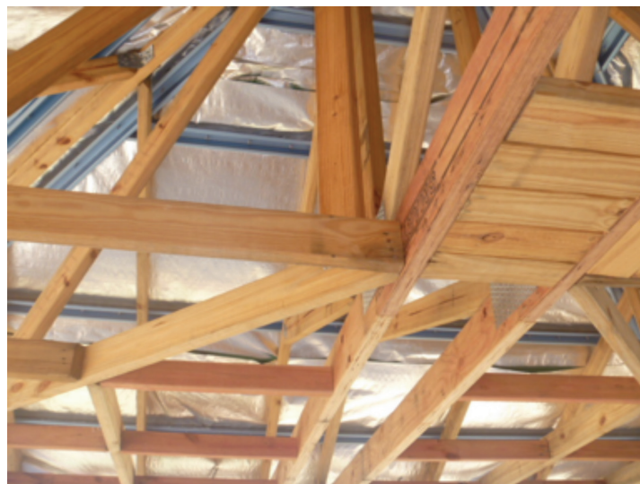
Photograph 8 – Inadequate connection of jack and hip trusses to girder truss in a C2 site
