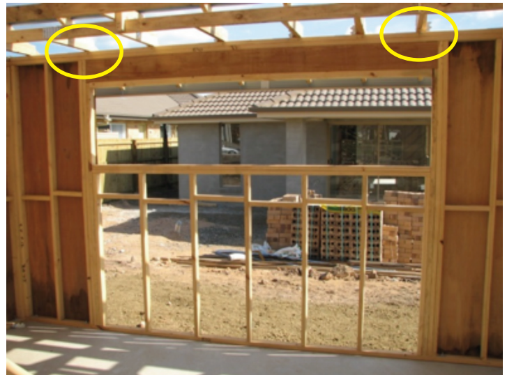
Photograph 11 – Plywood cannot be used to effect tie-down at sides of openings as the trusses highlighted above must have 300 mm min of ply to the right and left side respectively
