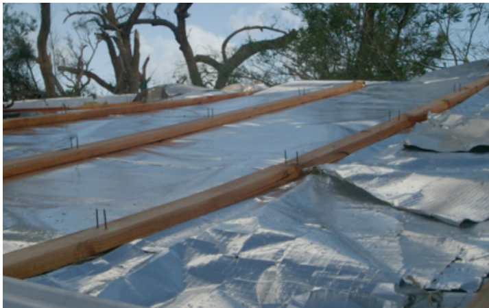
Photograph 5 – Roof sheathing and battens have failed due to nailed batten fixing where screws should have been used
