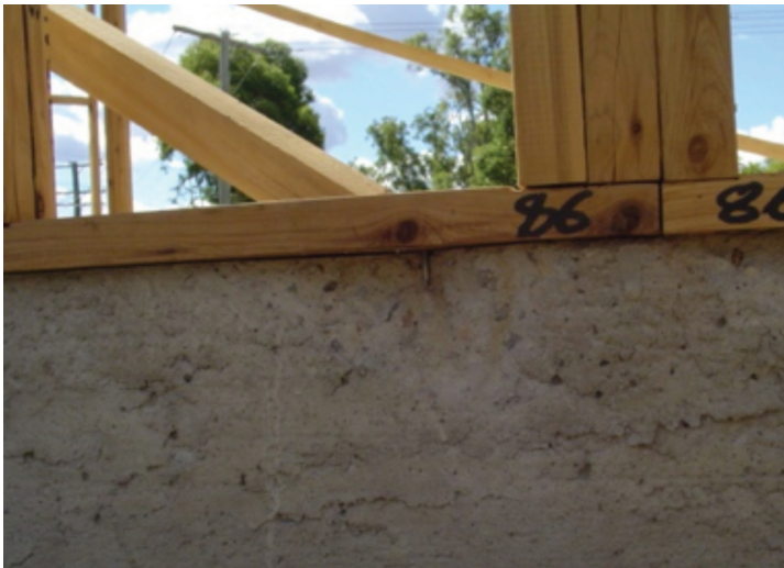
Photograph 13 – Nominal bottom plate connection compromised by excessive plate overhang
