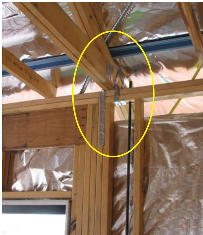
Photograph 7 – Double straps connecting girder truss to top plate and jamb studs (strap to jamb stud should have been centrally located on stud). Cyclone rod correctly located within 100 mm of truss tie-down
