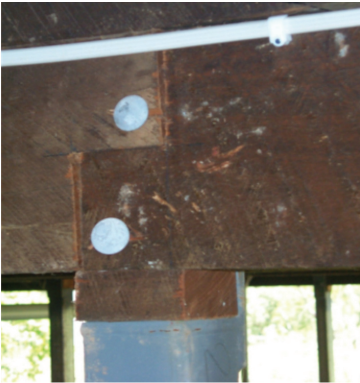
Photograph 15 – Minimum bolt end distances less than required to achieve uplift capacity. Also, unseasoned timber packer used is not suitable due to shrinkage
