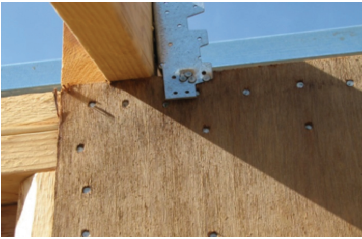
Photograph 2 - A structurally inadequate and incorrectly installed multi-grip. Nails too close to each other and edge of metal and also, too close to top edge of top plate
