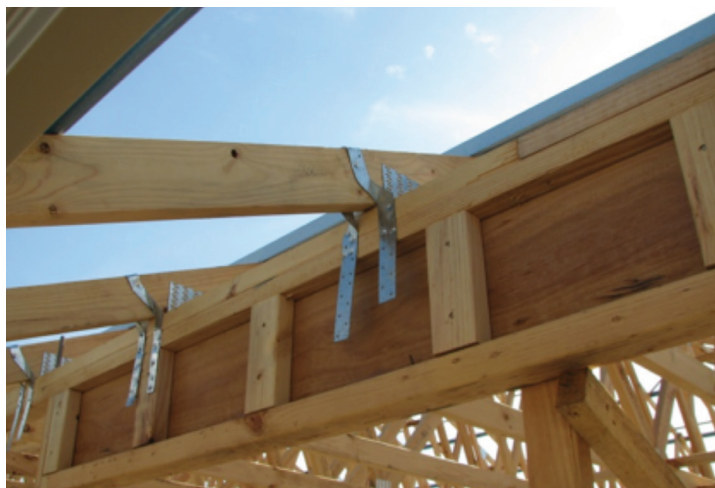
Photograph 9 – Incorrect practice for tying down over openings as top plates not tied to lintel
