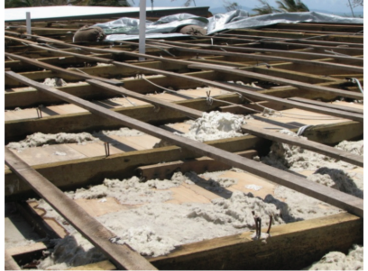
Photograph 4 – Roof sheeting 'blown' off due to inadequate fixing of the sheeting to the battens
